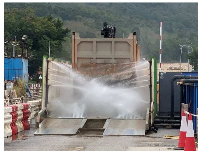
運泥車清洗設施 Wheel washing facilities for trucks
